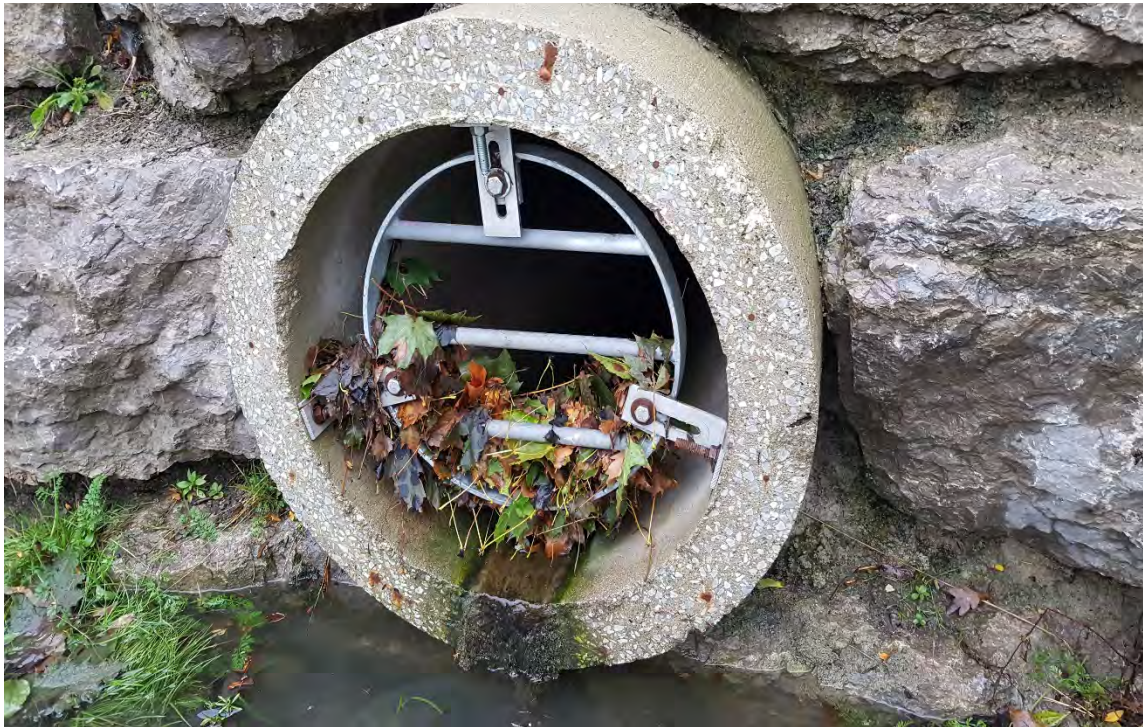
Photo 8 - Debris cover at inlet #2 culvert.
