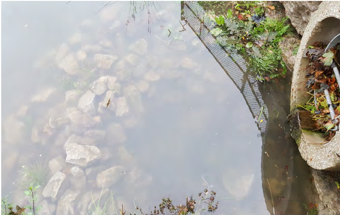
Photo 10 - Rock displacement at base of inlet #2 culvert.
