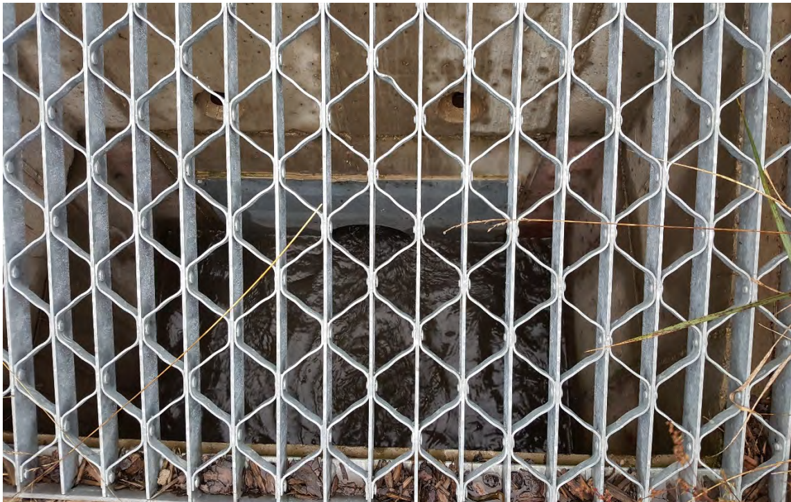
Photo 14 - Orifice plate on pond outlet.
