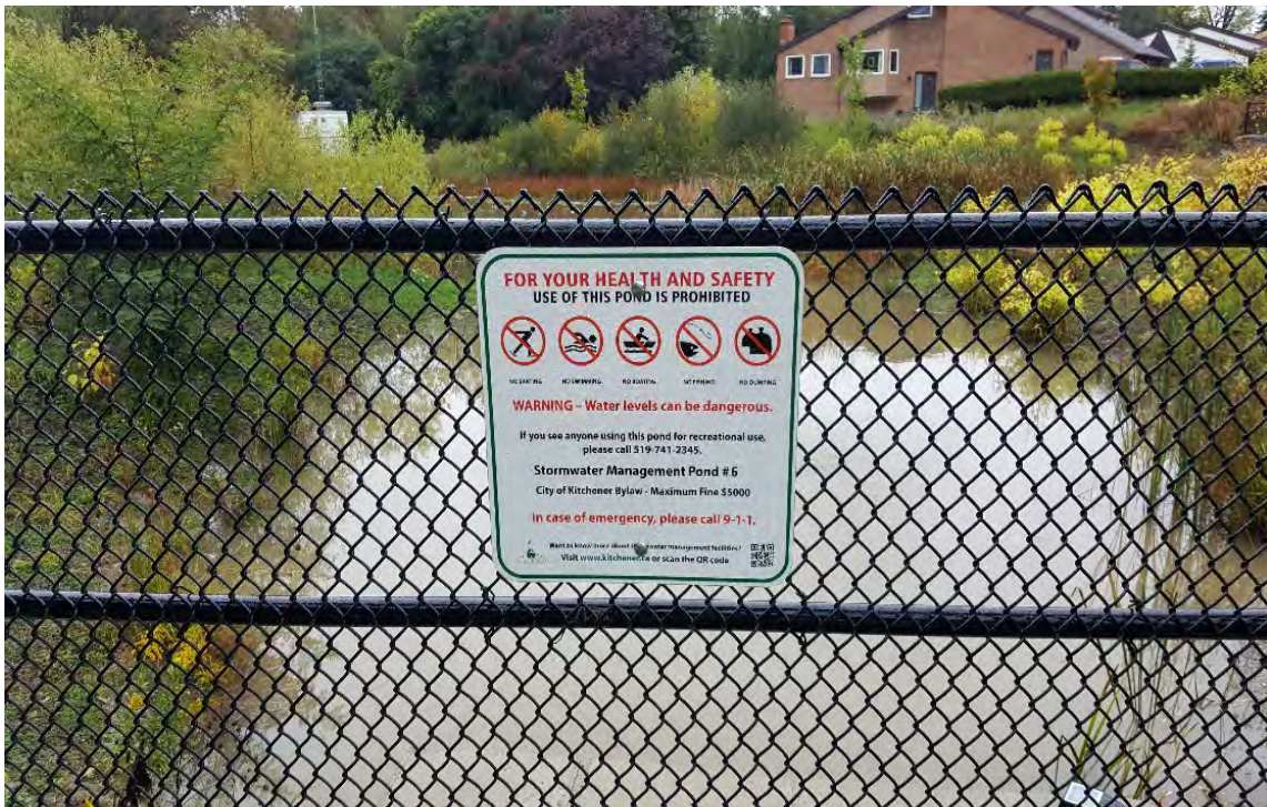
Photo 2 - City issued health and safety signage at inlet #1.
