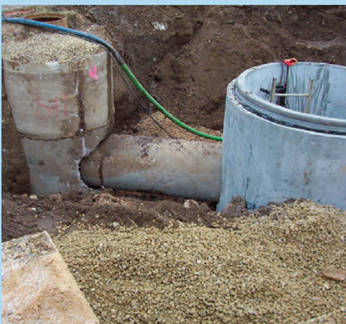
Oil and grit separator
