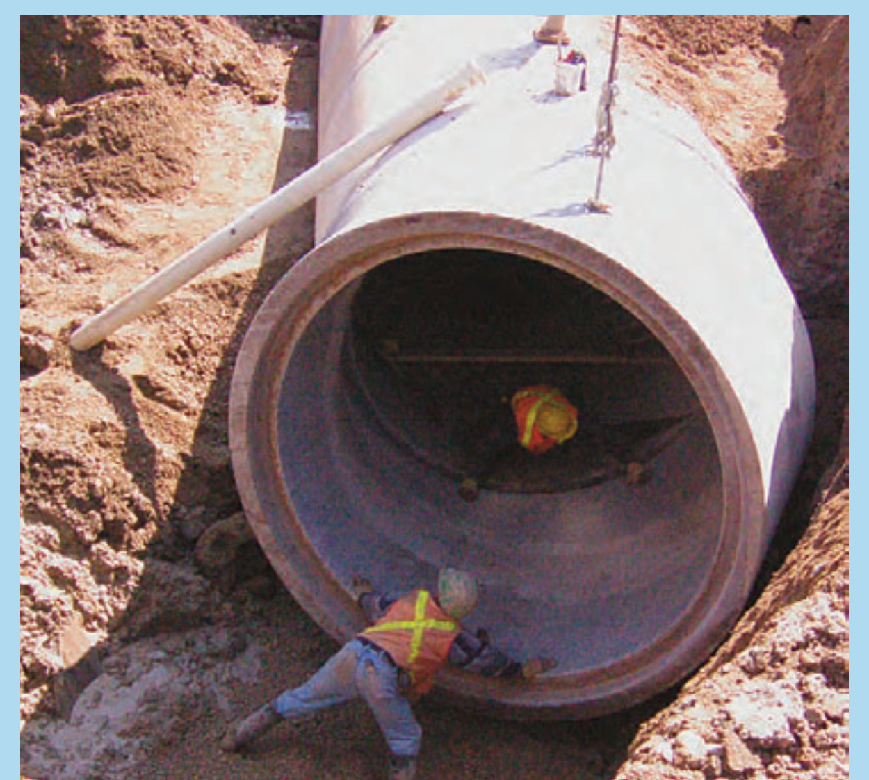
Orifice control / super pipe storage
